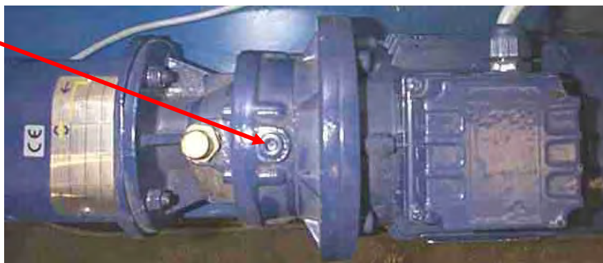
Figure 10 : Oil Separator Pump Gearbox
