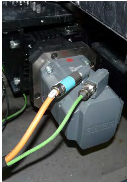
Figure 4 : Turntable Drive Motor Supply and Control Cable Plugs / Leads
