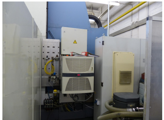
Back View / Electric Cabinet
